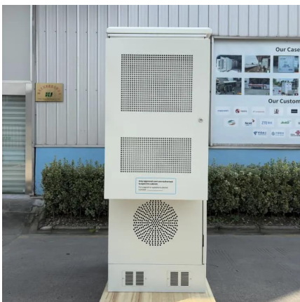
250kW ATEN Battery Energy Storage System , AGreatE
