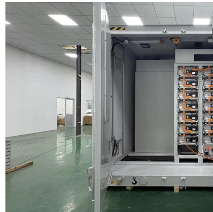
250 kW 575 kWh Battery Energy Storage System , Aggreko US
