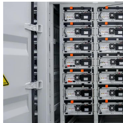
Energy storage container , SCU , energy ...
