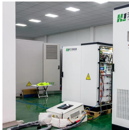
Container top photovoltaic energy storage system
