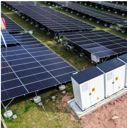
Solar Battery Container Systems: Scalable Power for ...
