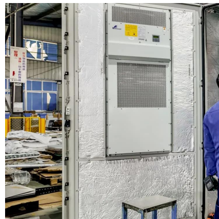
Sungrow deploys 60MWh BESS in 'one of Earth's harshest ...
