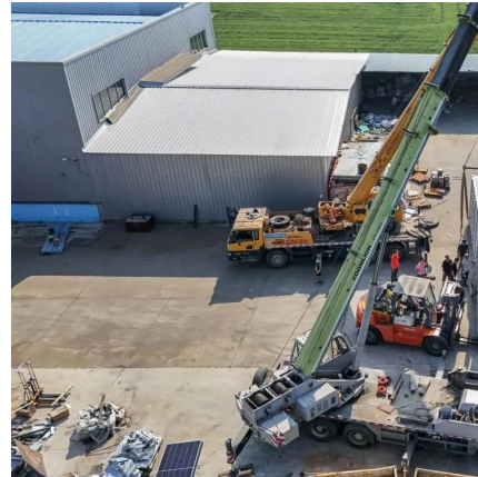
China's Sungrow deploys 60MWh BESS in Finland
