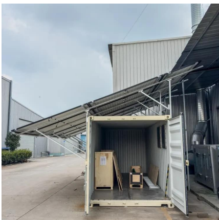
Containerised BESS Energy Storage Solutions , 0.5
