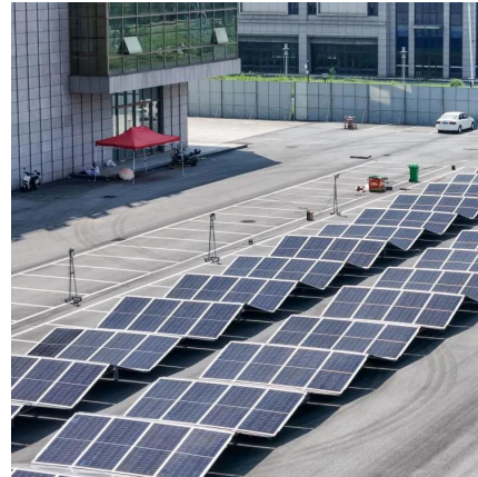
Utility-scale battery energy storage system (BESS)
