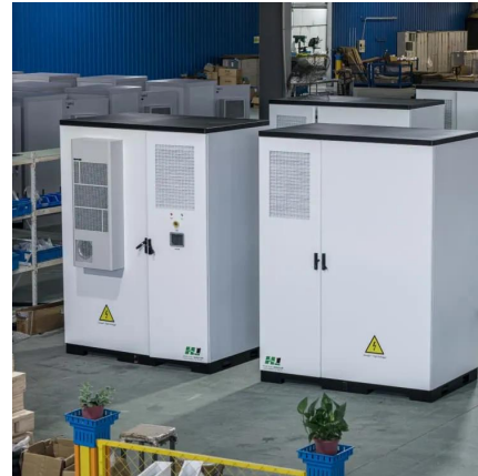
20KW Solar Energy Storage On the Container of the 40KWH ...
